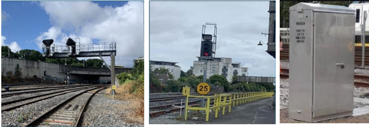
Figure 4-7 Typical Existing Signalling Infrastructure
