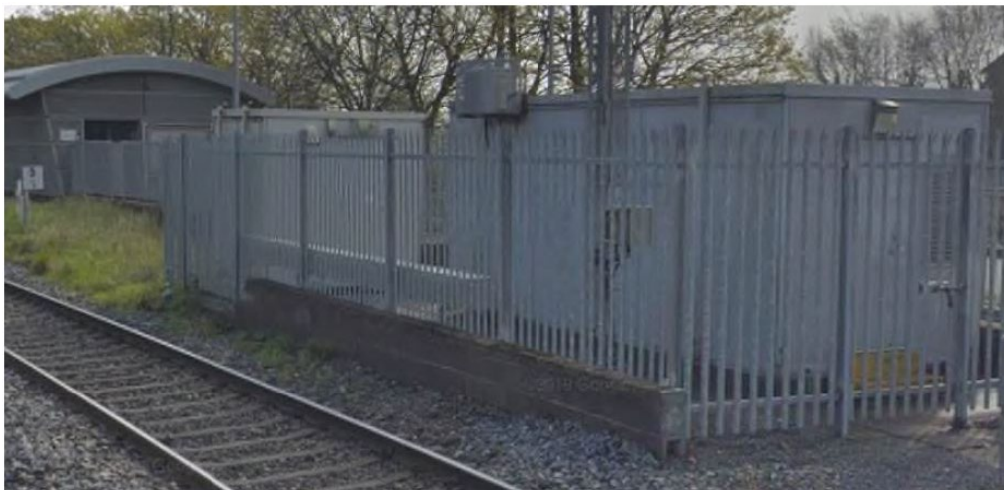
Figure 4-8 Typical Telecom Equipment Building
